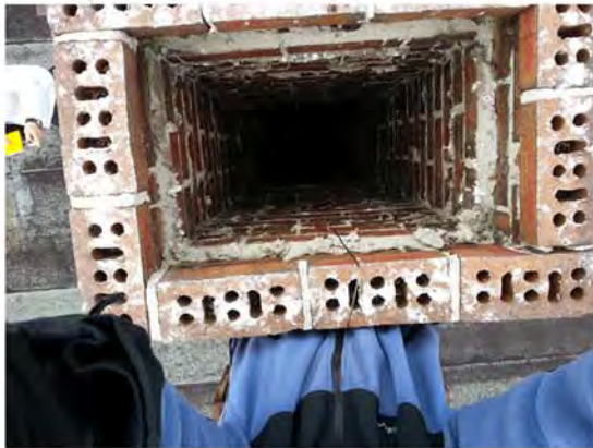
Interior chimney at Unity Christian High School on Burton Avenue
