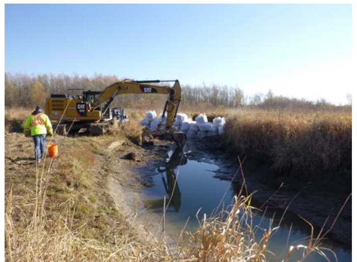
Below: repairing one of the breaches in the Mad River bank north of Sunnidale Concession 2
